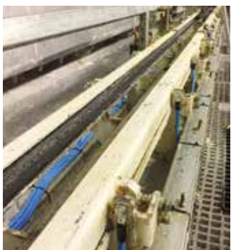
2 Cabling to earthing cabinet
