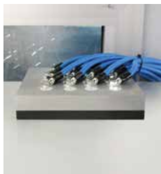
3 Connection to earthing cabinet
